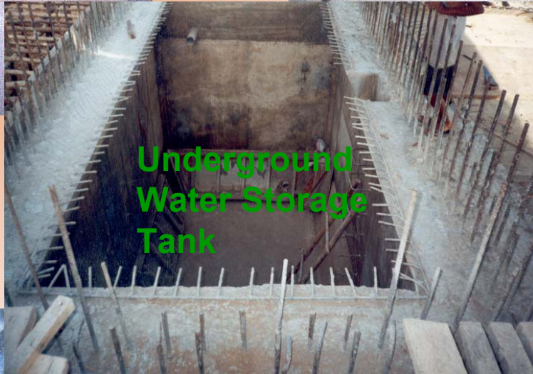
Ground Water Storage Tank
