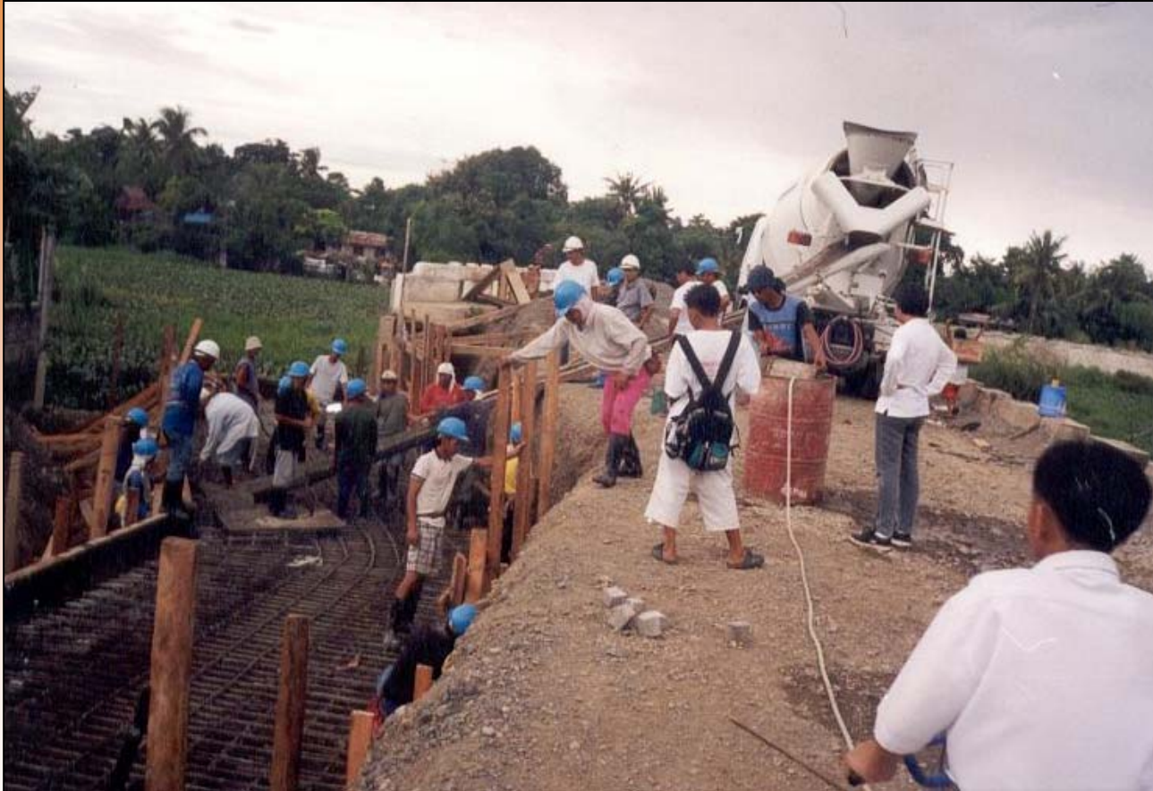
Construction of Interceptor Drains and Reinforced Concrete Box Culvert for the Comprehensive Drainage and Sewerage System of Cabanatuan City
